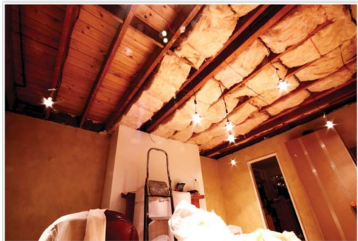
The Green Deal and other programmes encourage UK building owners to insulate lofts, among other efficiencies.
